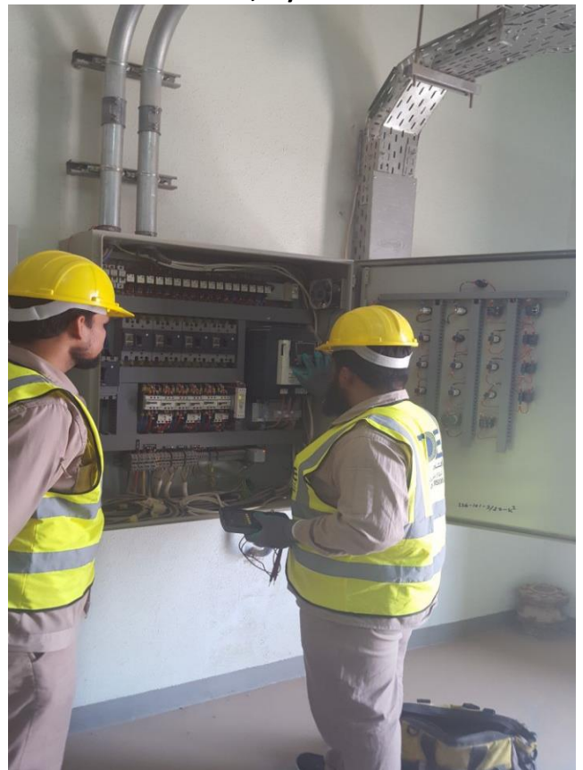
Inspection of Electric Panel Board for Fence light at Heliport-KAA, Riyadh
