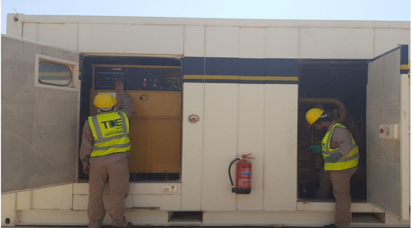
Generator maintenance at Heliport-KAA, Riyadh
