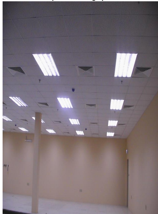
Dimmer Controlled Florescent Ceiling & Dimming lighting system for training hall.
