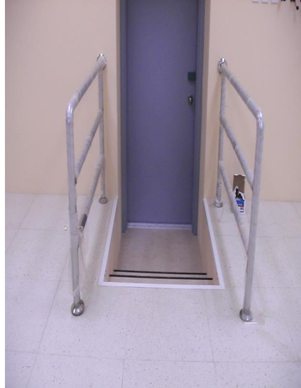
Raised floor steps and Railing System
