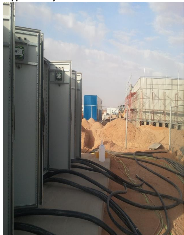
4MW ATS, Synchronization and Power Management system for temporary site
