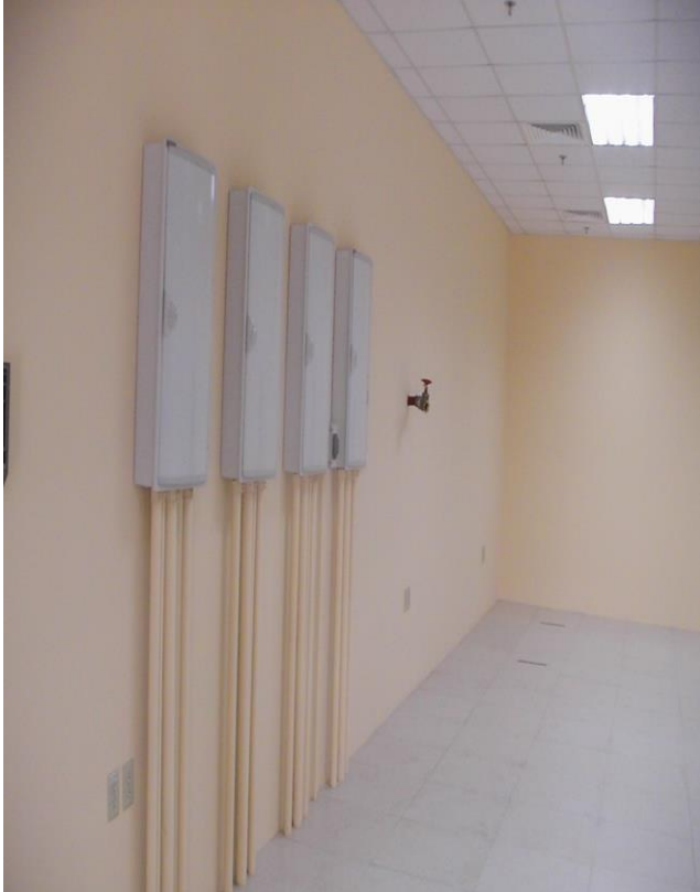
Dedicated Clean power supply panels for simulators.
